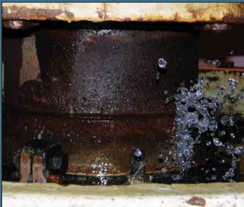
Leakage leads to equipment corrosion and premature bearing failure
