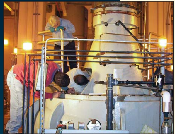
Unscheduled downtime and loss of production can be caused by conventional sealing methods.
