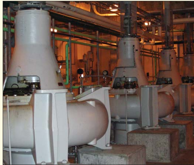
Effluent pumps, sealed with 8.00 inch (200 mm) diameter split seals, have been in service for over 12 years.
